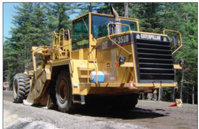
Figure 3.2 Pulverizing a failed asphalt pavement.
