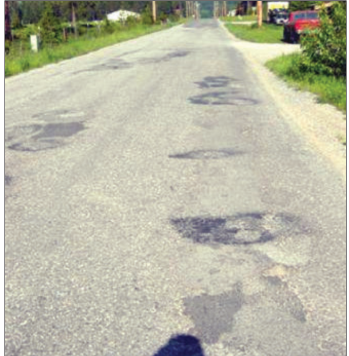
Figure 1.2 Excessive patching is often more expensive than FDR.
