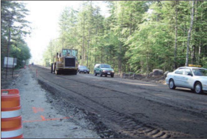
Figure 3.9 Traffic being allowed on completed FDR base prior to surfacing while processing operation proceeds in adjacent lane.
