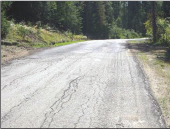
Figure 1.1 Example of pavement distress indicating base problems.
